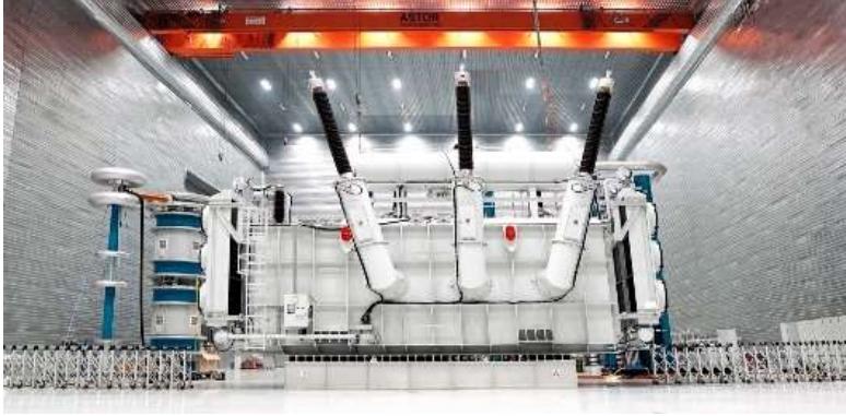
A section of the Astor Energy Test Laboratory
