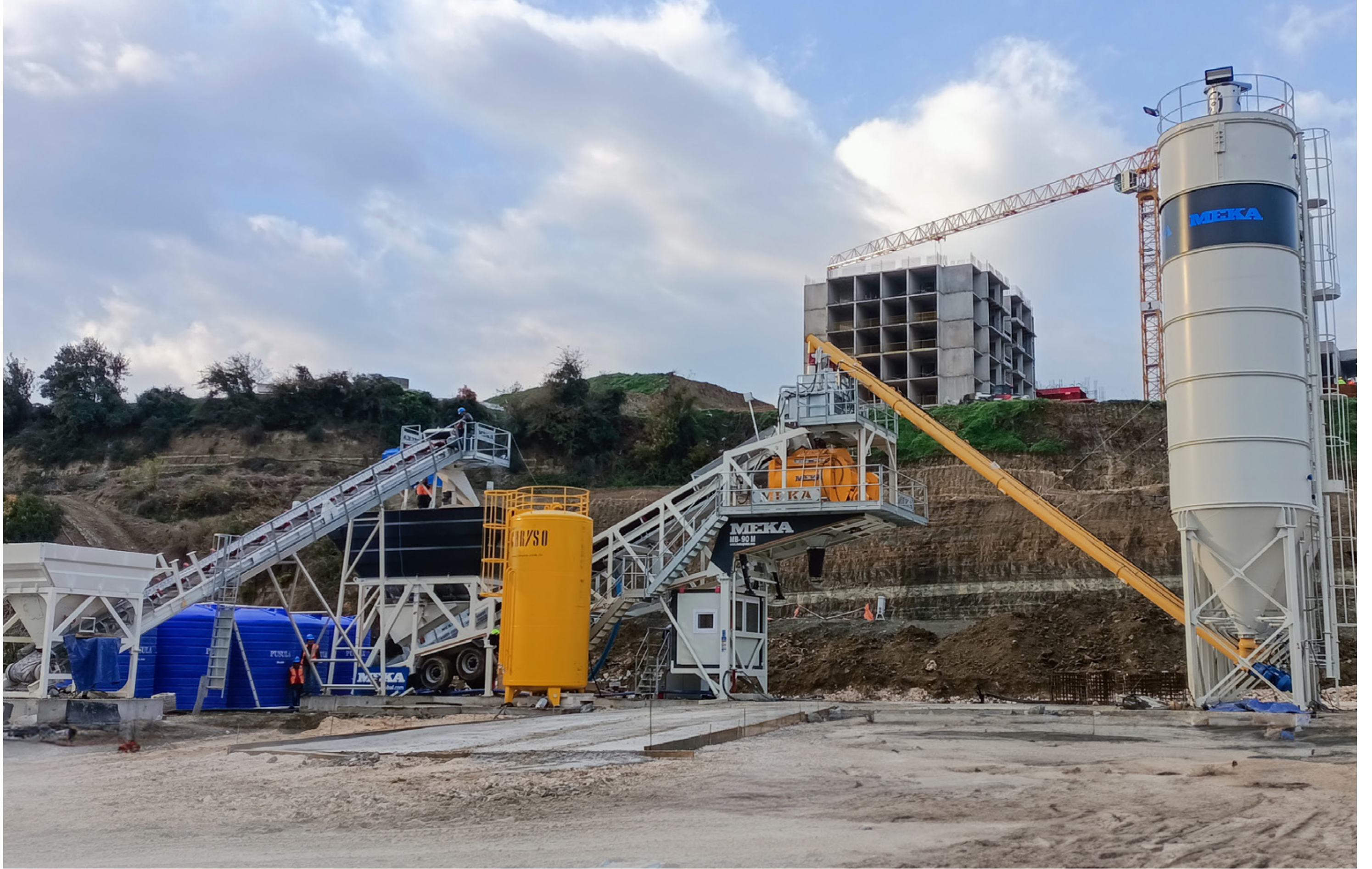
▲ MEKA Mobil Beton Santrali Hatay
