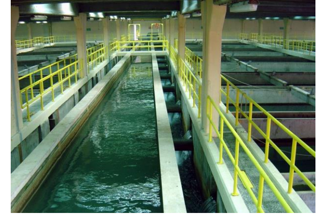
Ankara Water Treatment Project (Ankara)
