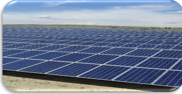
Larisa, Meterizi - 1 MWp
